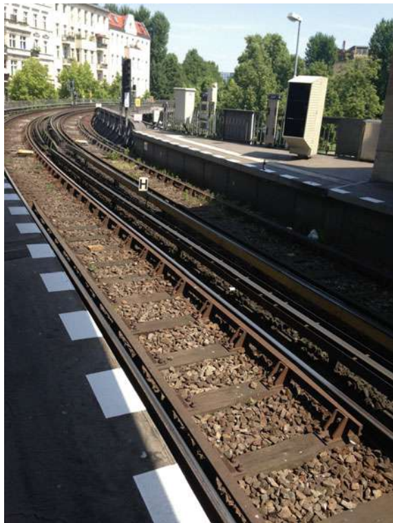
Fig. 3.18 Picture of third rail in metro operation. Source Author
